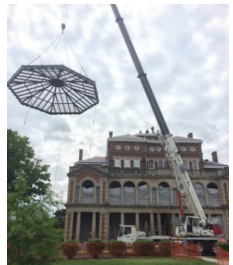
Top: Wasco's lightweight Horizon S-Series system bathes the vestibule in natural daylight. Below: The crane lifts the single piece structure.
